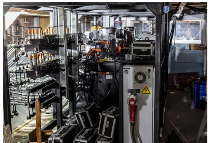
Below: 48-point plc motion control system
