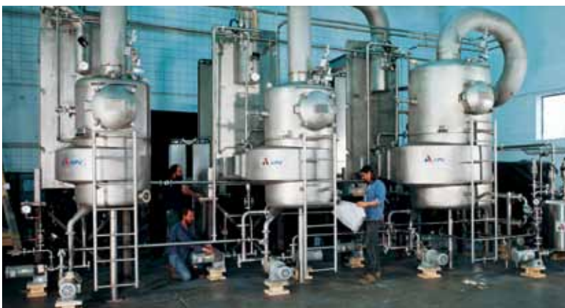
Figure 13. Plant representation. Triple-effect Falling Film Evaporator system followed by a double-effect forced circulation tubular finisher. A distillation essence recovery system was provided to recover the key essence components from the juice and in particular the methyl anthranilate.
